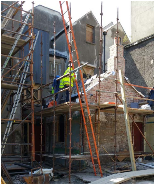
Rear view of no.16 with weathering in place and annexe roof being slated. (Photo: P. Walsh)
