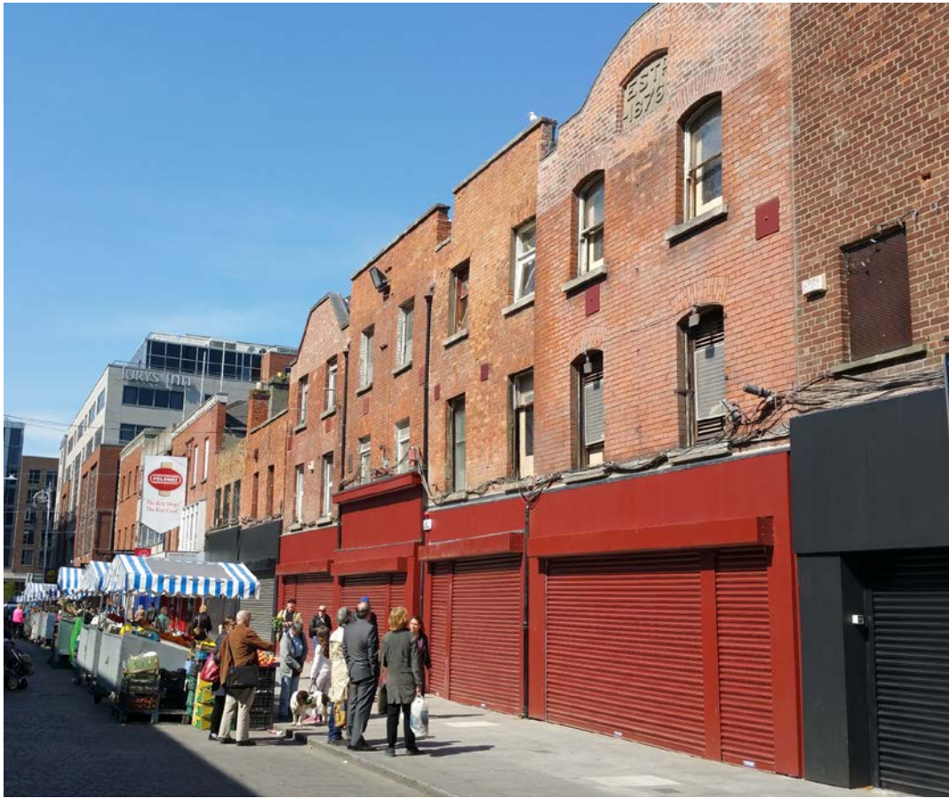
Front facades minus hoarding. New roller shutters in place. (Photo: P. Walsh)
