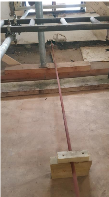
Internal steel tie (Photo: J. Donnelly)
