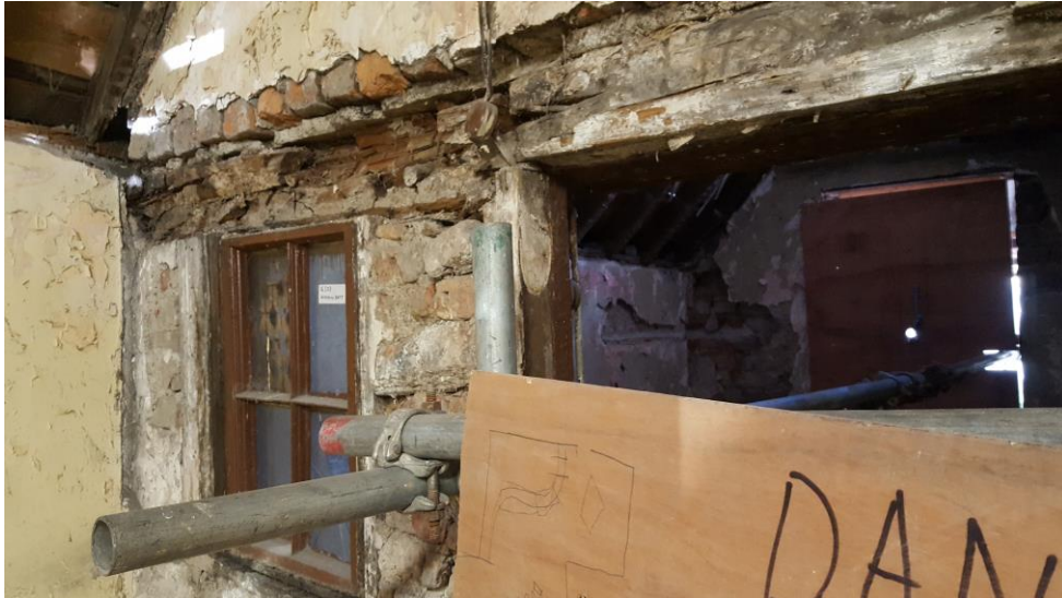
Decayed timber lintel in internal partition wall (Photo: J. Donnelly)
